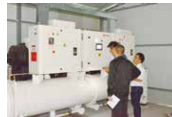
Rotary liquid chiller
