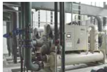
Rotary liquid chiller
