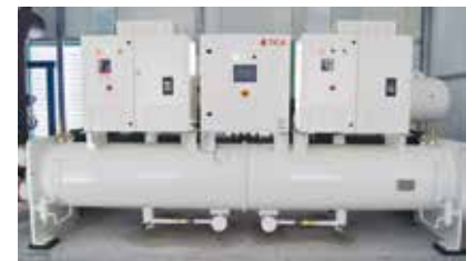
Rotary liquid chiller
